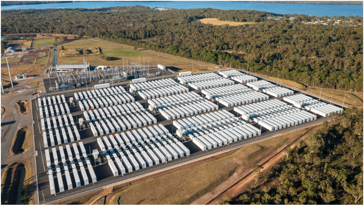
Waratah Super Battery, New South Wales
